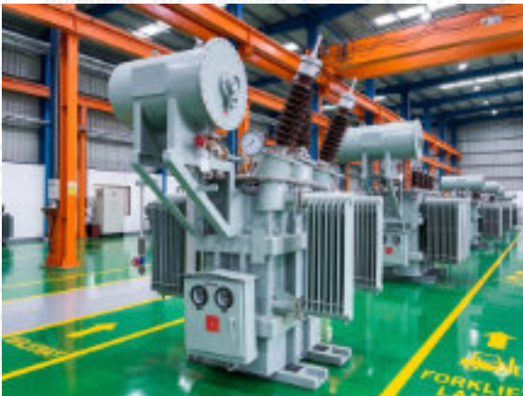
500 KVA 66 kV supplied to Zambia
