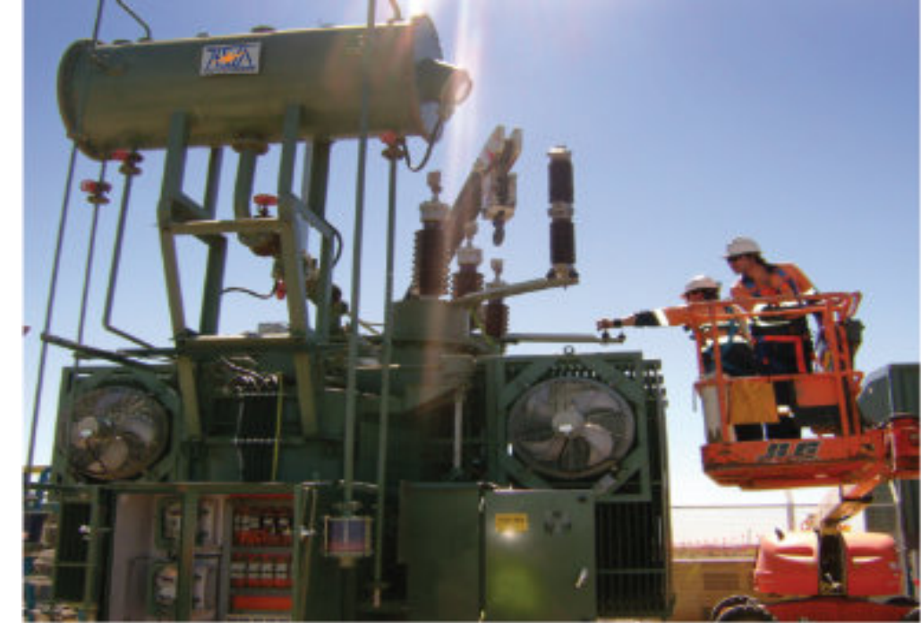
12.5 MVA, 66 KV Transformer Supplied to Australia.
