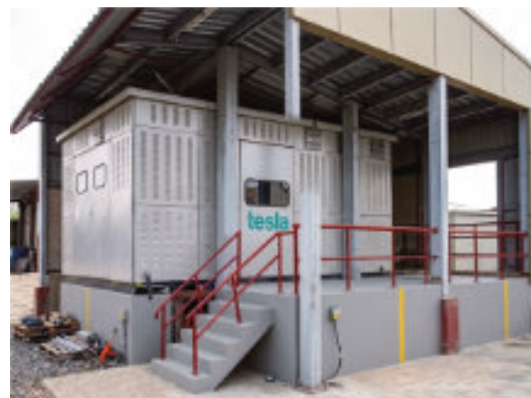
2500 KVA 33/0.433 KV USS with Cast Resin Transformer and GIS installed at a Shopping Mall .
