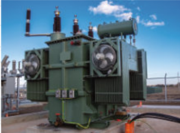
12.5 MVA 66 kV supplied to Australia
