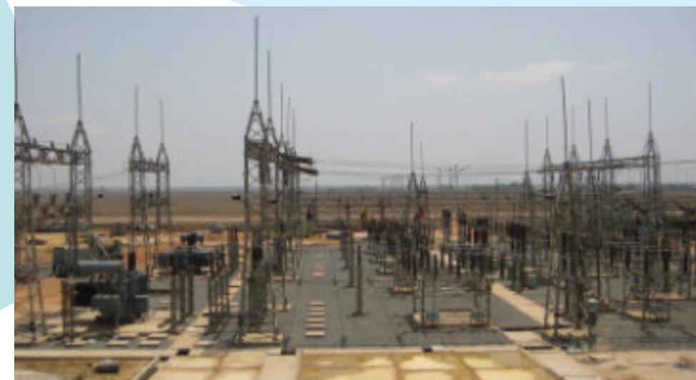
132 kV Switchyard Commissioned in 2025-26
