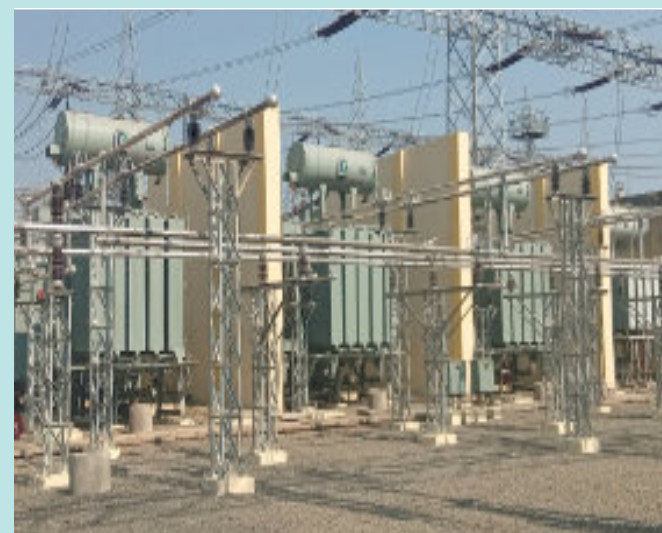
400 kV Substation Commissioned in 2025-26
