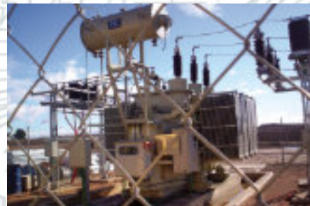
10-12.5 MVA 66-20KV UTE SOLAR-SS to Spain .
