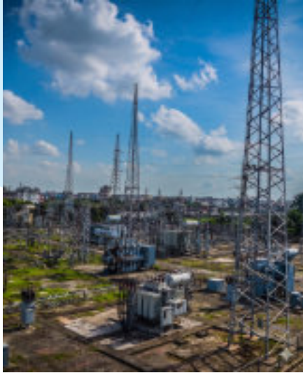
33 kV Substation Bangladesh
