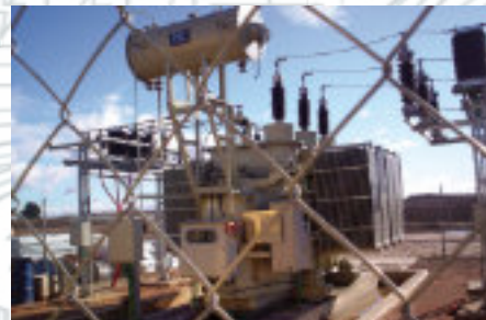
10-12.5 MVA 66-20KV UTE SOLAR-SS to Spain .
