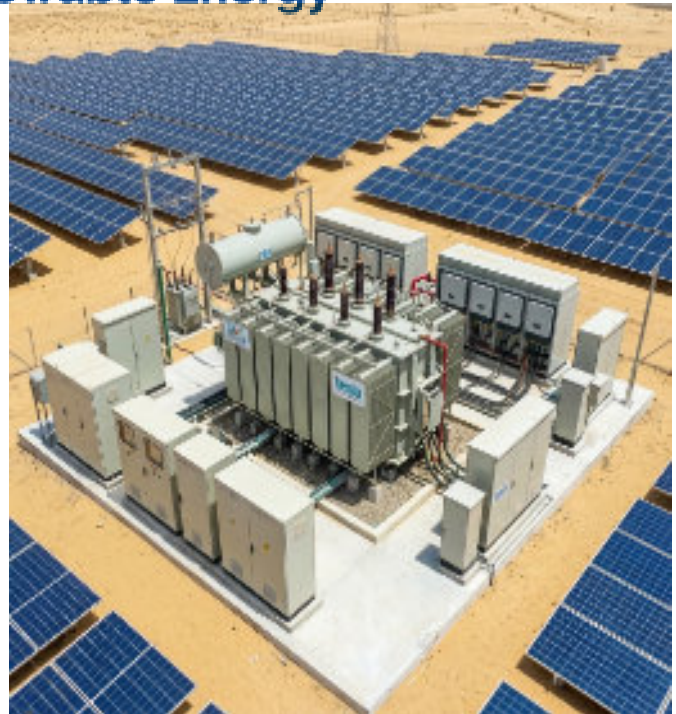
12.5 MVA 33 x 0.660-0.660-0.660-0.660 kV
