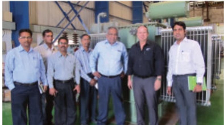
NEPEAN POWER MD's visit & testing of 10 MVA 66 KV Transformer
