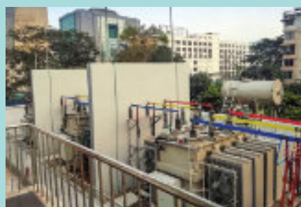
20/28 MVA, 33/11 KV Power Transformer supplied to DESCO Bangladesh .
