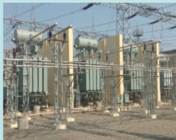
400 kV Substation Commissioned in 2025-26
