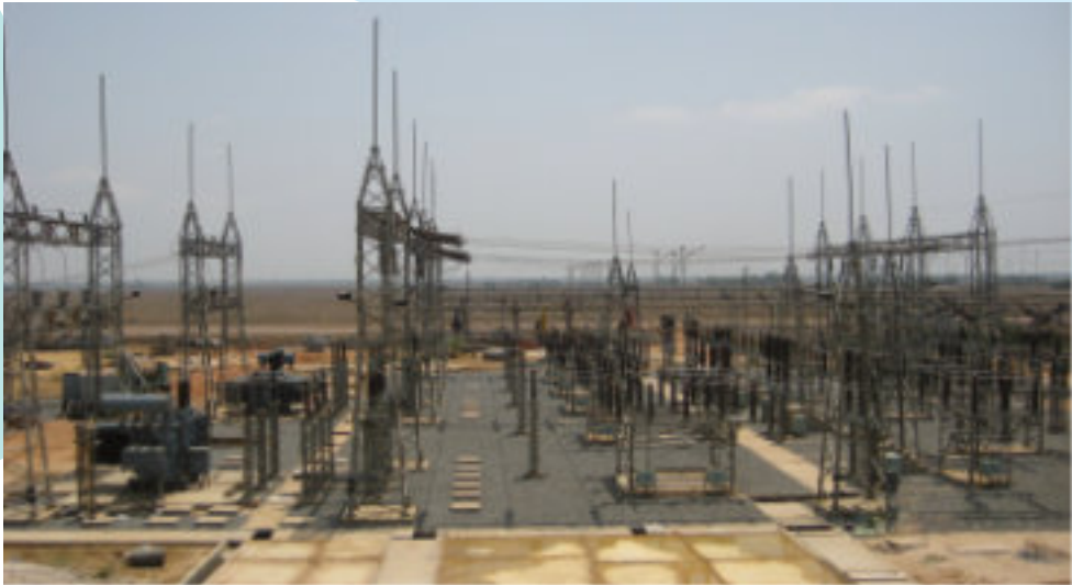
132 kV Switchyard Commissioned in 2025-26
