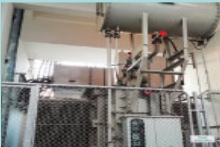
28/35 MVA, 33/11 KV Power Transformer supplied to DPDC Bangladesh
