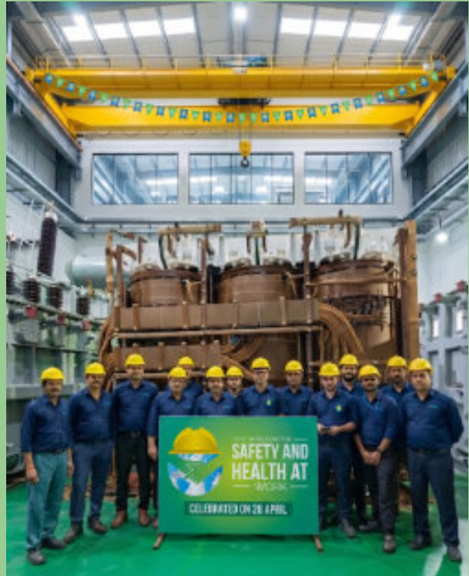
50 MVA-132kV CC Assembly
