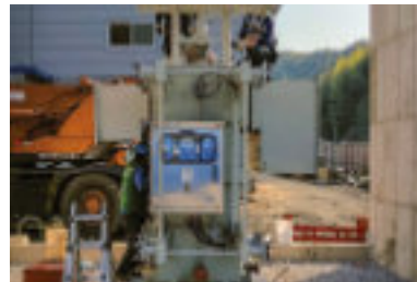
1.6 MVA, 10.5/0.46 KV, 60 Hz. Auxiliary Transformer Supplied to South Korea.
