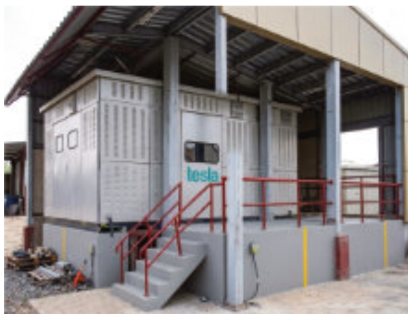
Tesla supplied 2500 KVA 33/0.433 KV USS with Cast Resin Transformer and GIS installed at a Shopping Mall .
